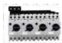
MMSs with bus bar connection
